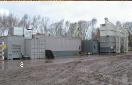
The new Biojoule processing and pelleting plant has the capacity to produce 10,000 tonnes of pellets a year. The plant is totally self-contained and designed so that all the heat is captured and recirculated through the wood chip powered drying unit.
